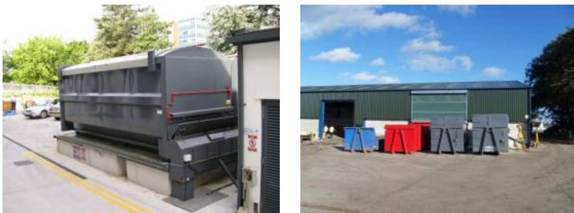
Figure 18 - Hook bins at boiler and in depot
